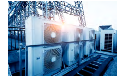
HVAC and Building Systems
