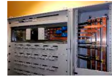
Electrical Distribution and MCCs
